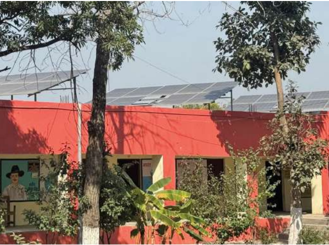
Rooftop Solar Power System Installed at one of the schools
