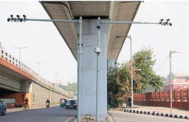
ITMS installed at one of the junctions at Delhi
