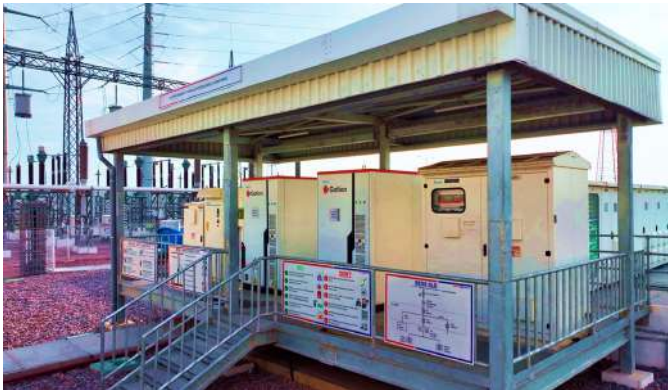
Battery Energy Storage System (BESS) at Kharkhoda, Haryana
