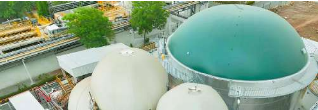
A view of biogas plant installed at Manesar facility
