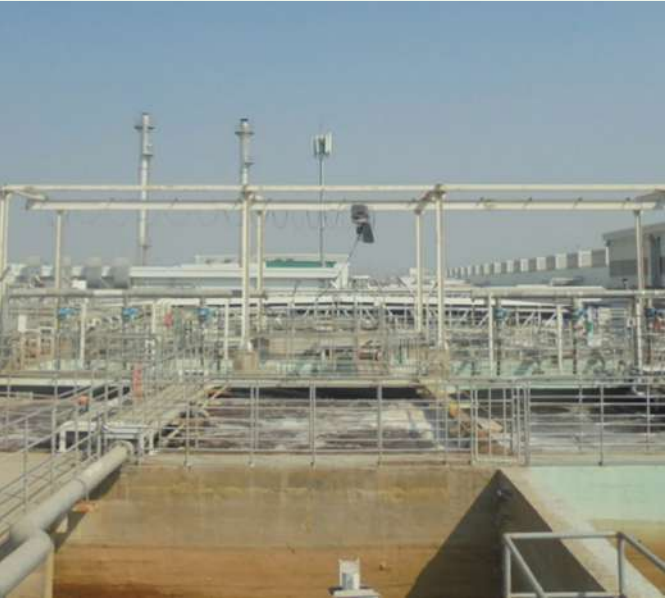
Hansalpur ETP Plant
