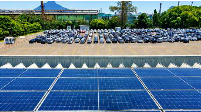
A view of rooftop solar power plant installed at RPDC Bengaluru
