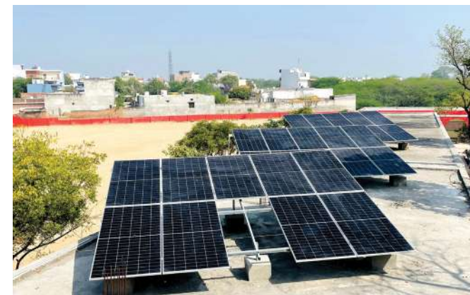
Rooftop solar power system at one of the government schools supported
