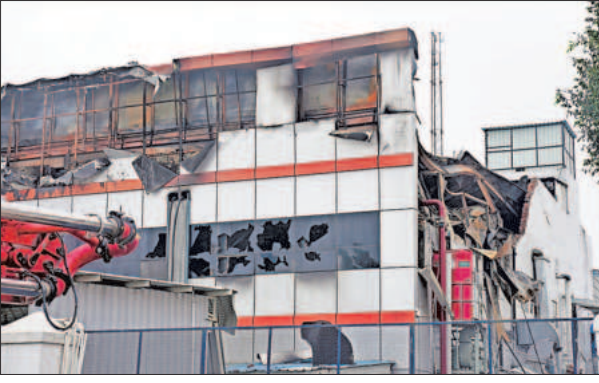
The firefighters were dousing the flames when a wall and iron beam at the unit collapsed. ABHINAV SHAHA
