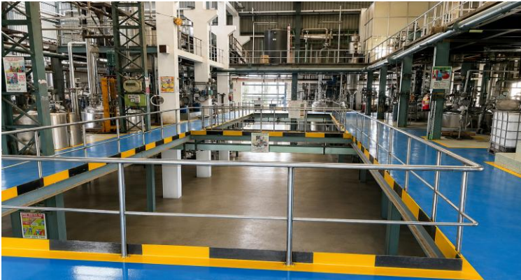
Patancheru, Telangana Chemicals Manufacturing
