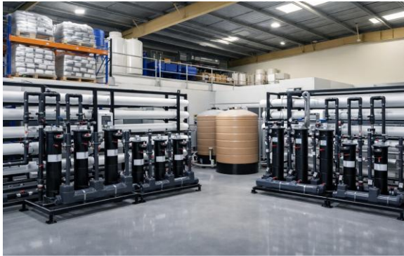
UAE Assembly Unit, ICV Certified Facility
