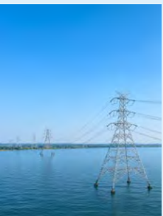
765 kV AHMEDABAD- NAVSARI D/C TL, GUJARAT, INDIA
