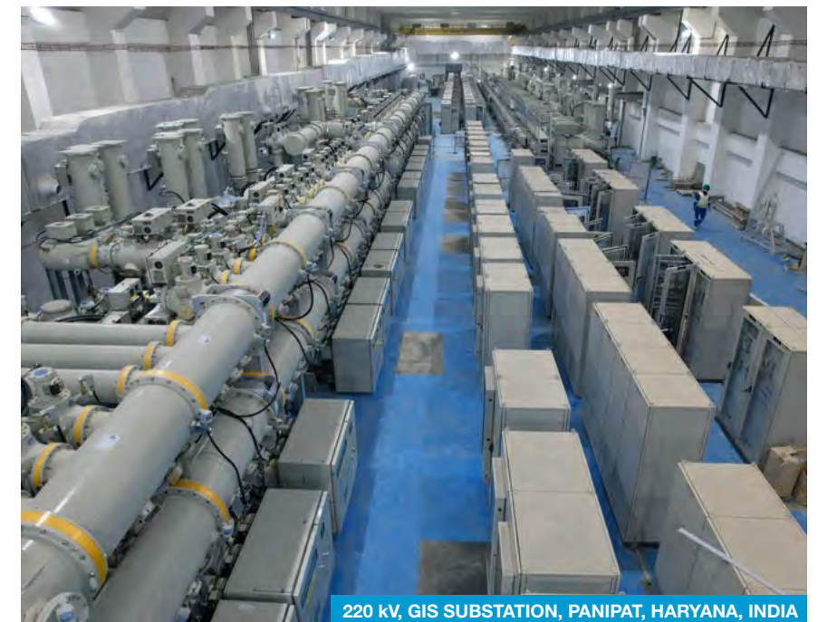
220 kV, GIS SUBSTATION, PANIPAT, HARYANA, INDIA
