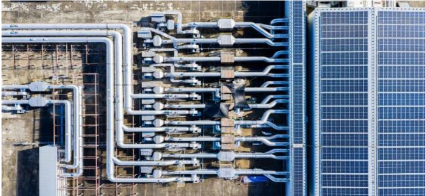
Sustainability Project for Energy Performance Improvement for Complete HVAC system for MNC
