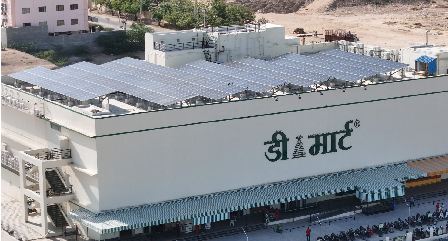
Rooftop Solar Panels
