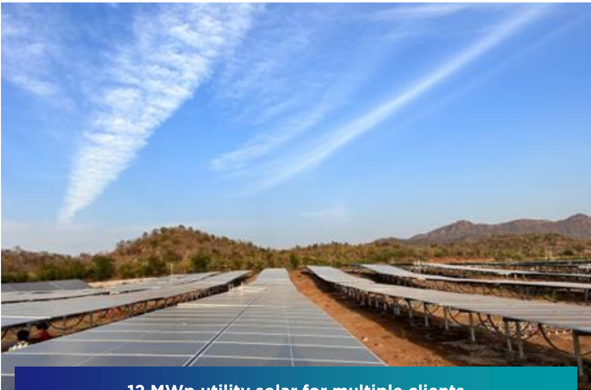
12 MWp utility solar for multiple clients
