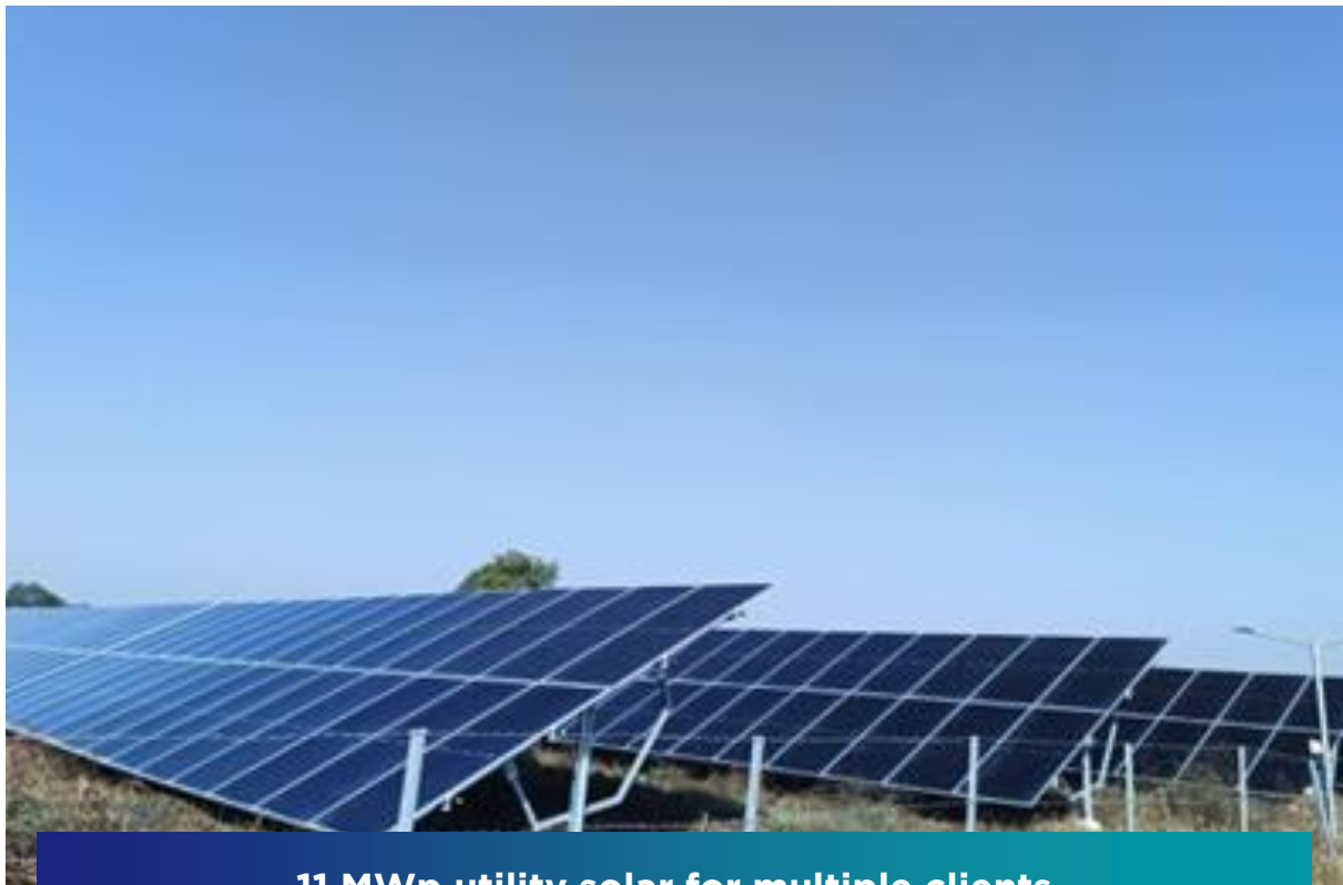
11 MWp utility solar for multiple clients
