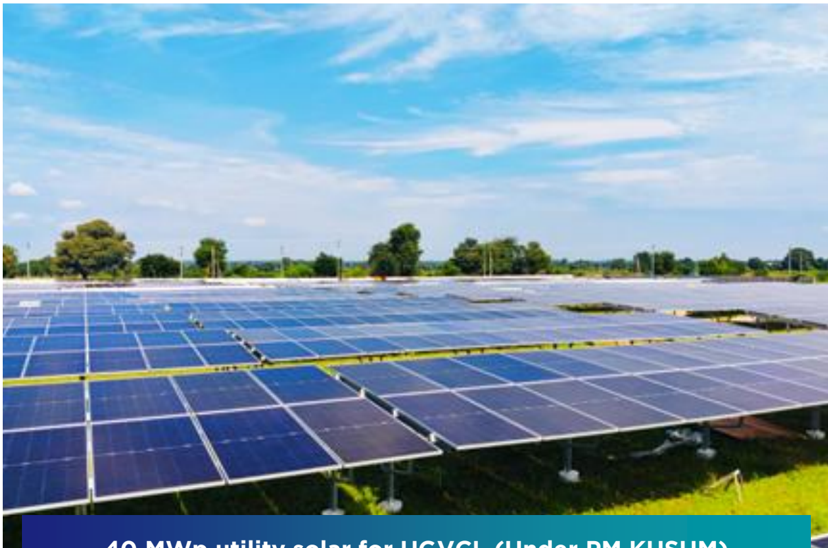
40 MWp utility solar for UGVCL (Under PM KUSUM)
