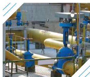
City Gas Distribution
