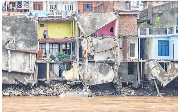
Houses are seen damaged in the aftermath of torrential rain-triggered landslides and flash floods, in Rajouri district, Jammu and Kashmir
