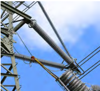
Pole with Insulated Cross-Arm
