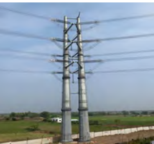
Twin Pole Structure
