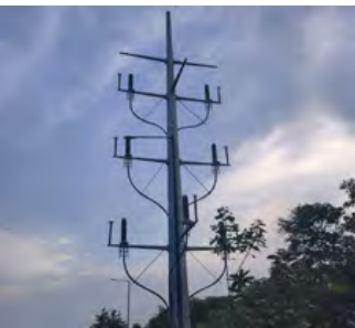
Cable Termination Pole
