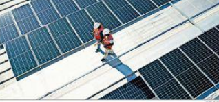
The electricity generated will be supplied to state-owned SJVN under a 25-year power purchase agreement at a tariff of ₹6.74 per unit, providing long-term revenue visibility.
